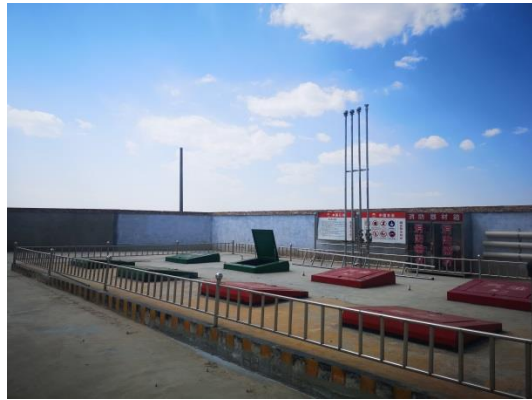
储罐区排空阀
