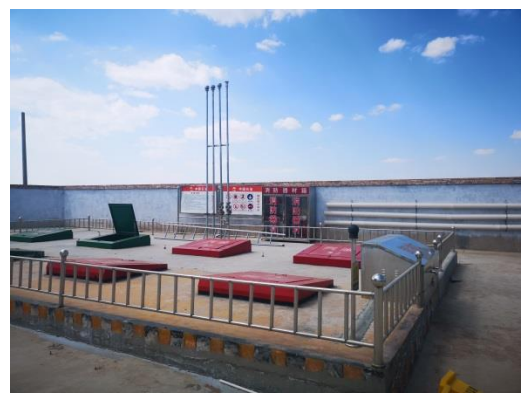
储罐区排空阀
